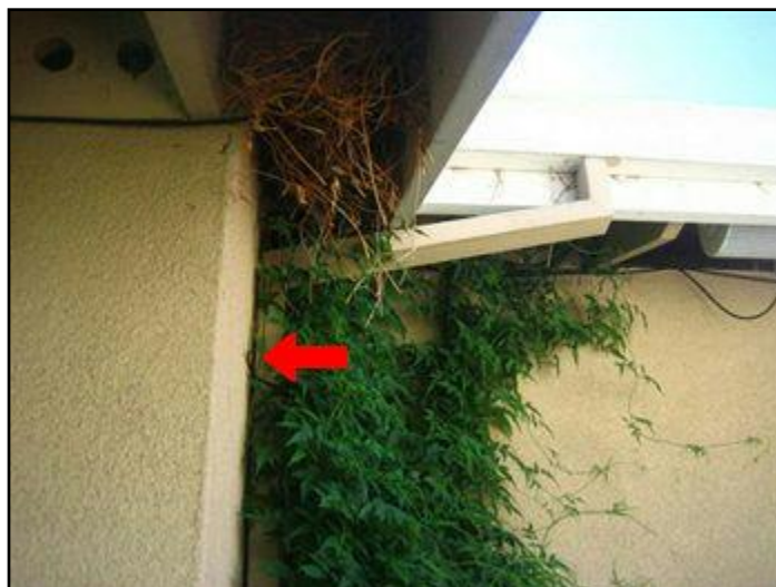
4. Trees or shrubs too close to building
