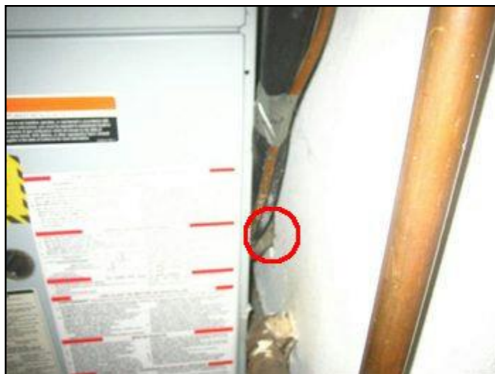
10. Sealing needed at fire separation wall
