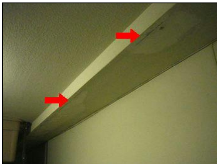
6. Water stain(s) noted
