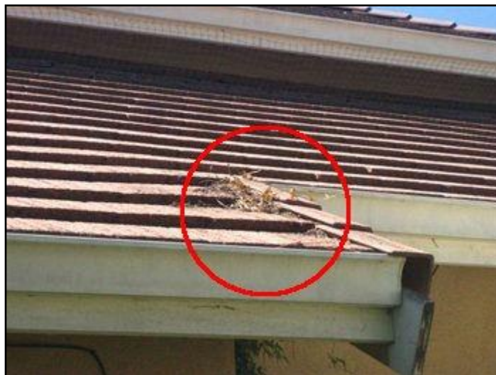
1. Debris present on roof
