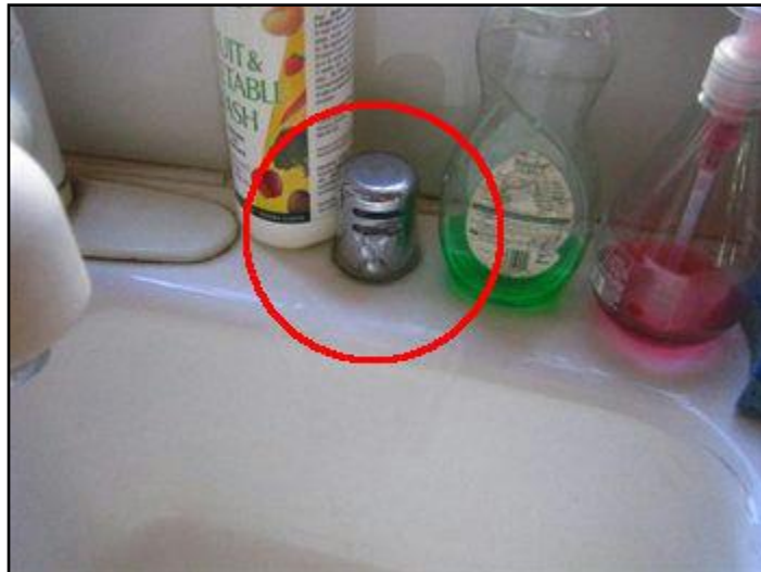
11. Backflow prevention defective
